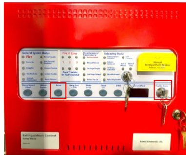
Figure 30: Fire Alarm Control Panel Interface
